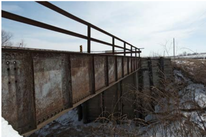
Many problematic bridges are owned by counties or municipalities and are load restricted or closed altogether, which means a journey from the farm to the local elevator becomes a 30-mile trip verse a 10-mile trip. Photo by Joe Murphy
