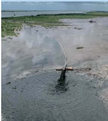
Once material and water from the bottom of the Mississippi River is dredged, it discharges nearby, which creates additional marsh habitat for the local ecosystem. Photo courtesy of Big River Coalition/P.J. Hahn
